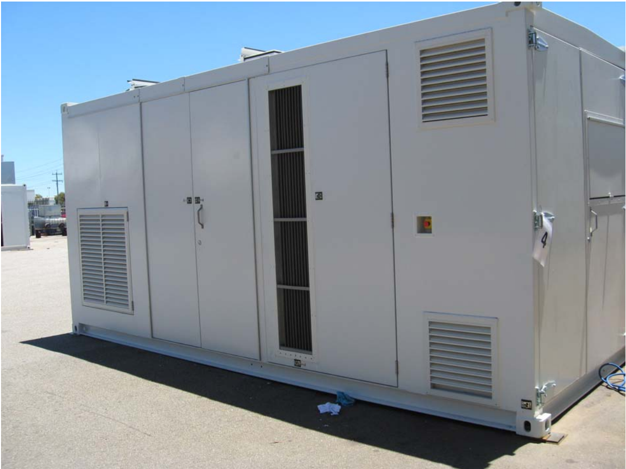
Moisture Eliminator Which has been installed on an Acoustic Enclosure
